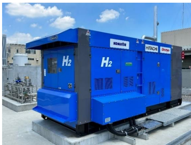
Hydrogen-light oil mixed combustion Generator delivered Komatsu Oyama Plant
