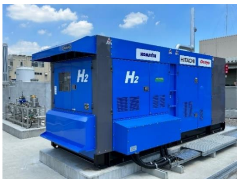
A hydrogen co-firing power generator introduced by Komatsu's Oyama Plant.
