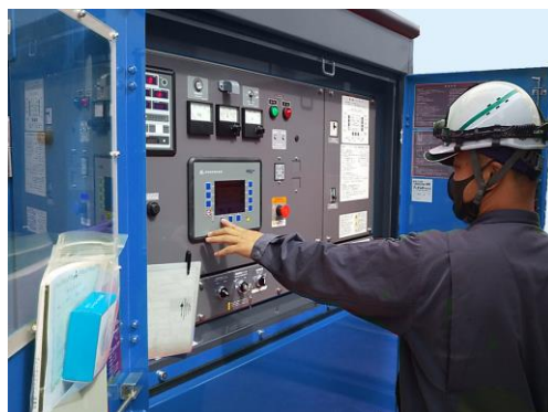
Test run inspection at delivery of a generator
