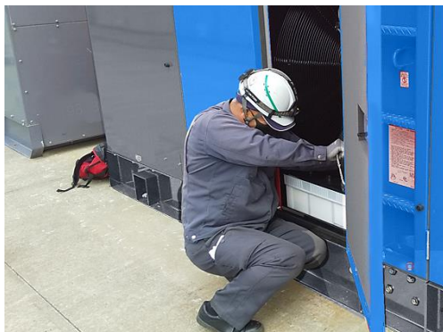
Machine internal inspection at delivery of a generator
