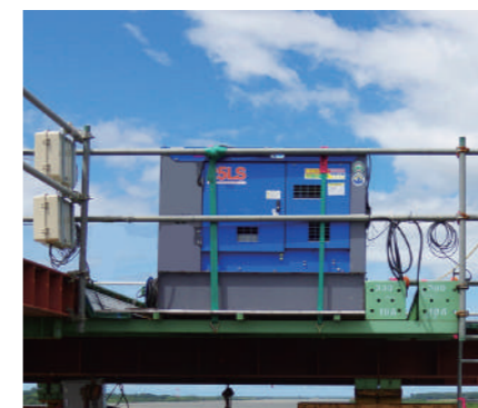
Power supply for a construction site (Japan)
