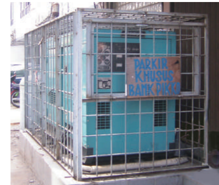
Backup power supply for bank (Indonesia)
