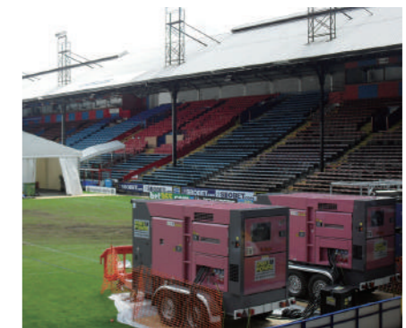
Temporary power supply for an outdoor festival (UK)
