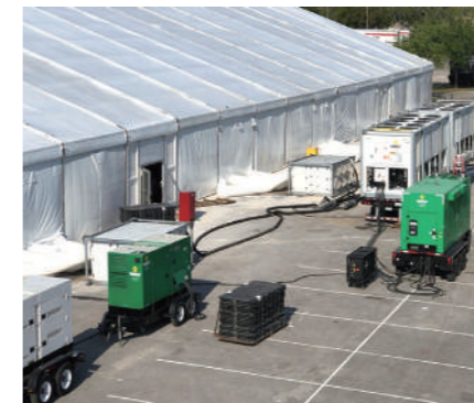
Temporary power supply at a vaccination site (US)
