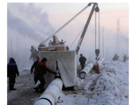
Power supply at a petroleum pipeline construction site (Russia)
